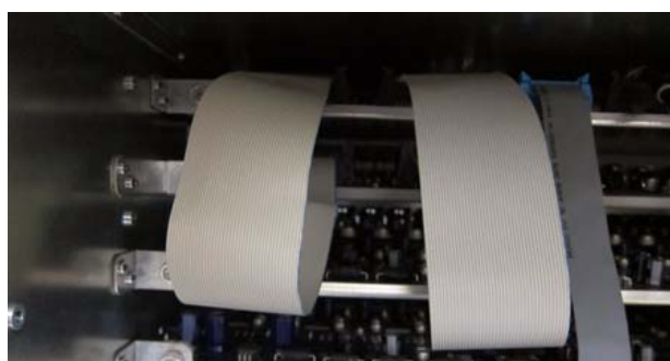
IOx ribbon cables connected to FOH IO card
