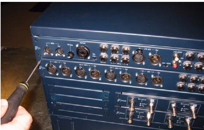
Securing the IOx card to the back panel of the FOH Rack
